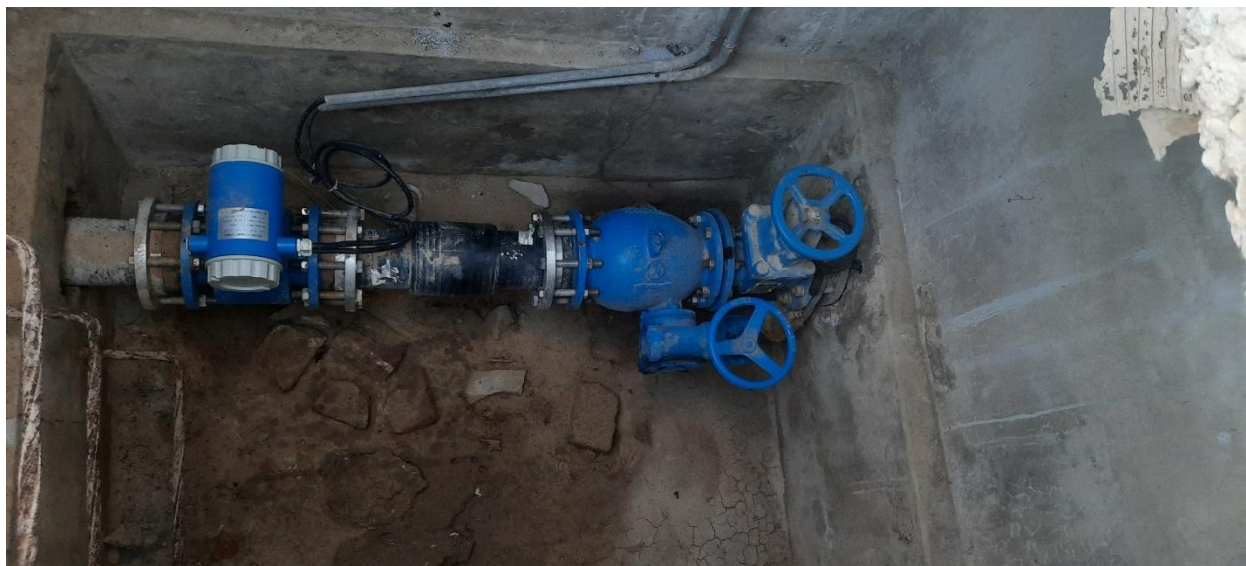
Mine water injection pump at Meghay Jo Tar
