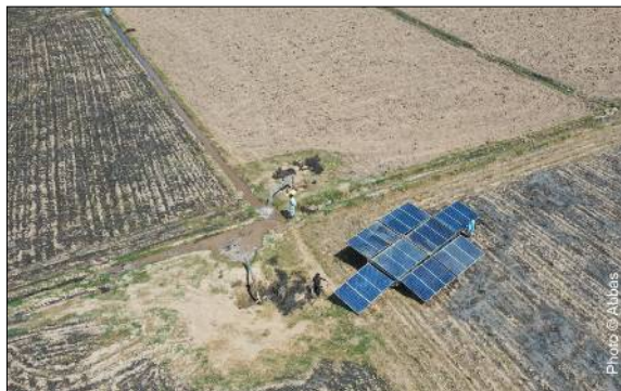
Figure 5: Solar power for tube wells in Rajanpur, Punjab.
