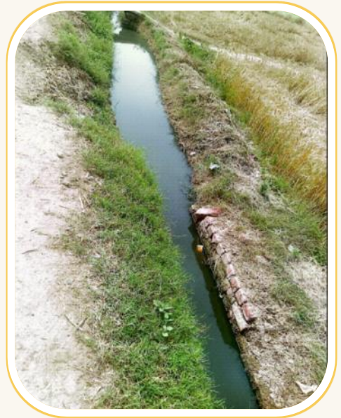
Sewerage water in streets and fields is a common scene in Chak No. 76/5-R
